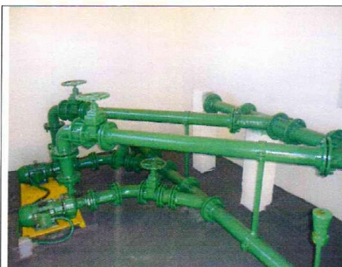
Conjunto Moto-Bomba - EAT 11 Booster
